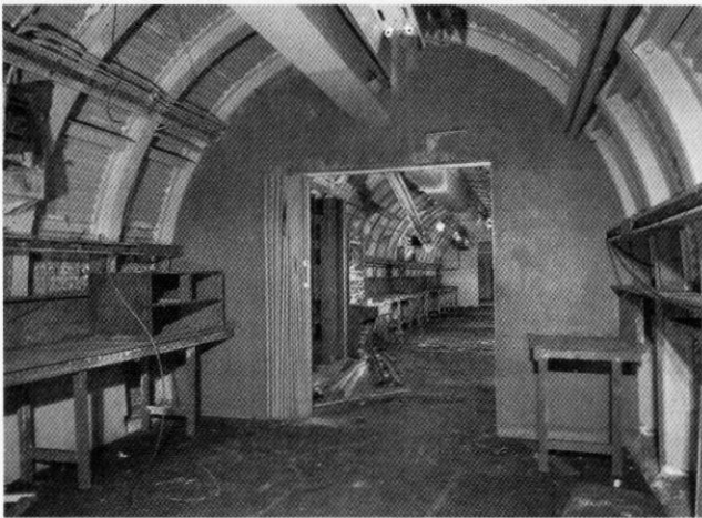
Room 45, Teleprinter Room. Viewed from room 30 through the folding doors. A GPO 10 x 40 PMBX switchboard and equipment racking can be seen on the left with operator benches beyond. Photo by Nick Catford
